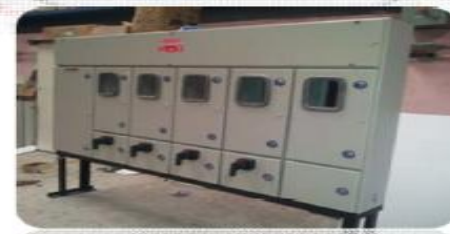
EB Metering Panel
