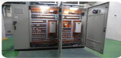
VFD Panel with Bypass & PLC
