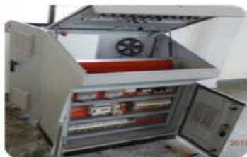
Control Desk Panel
