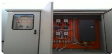
Chiller Compressor Panel
