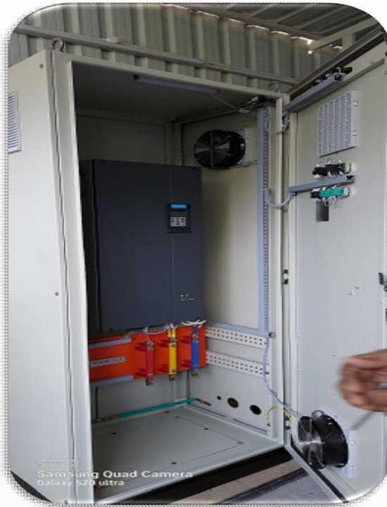
132KW INOVANCE VFD- RST CRUSHER- GUMMUDIPOONDI
