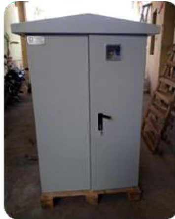
CHILLER VFD PANEL
