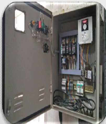
STRIDES SHASUN-AHU VFD PANEL
